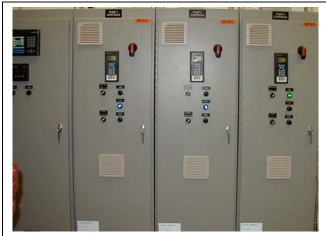
PLC Control Panel with Three 15hp VFD cabinets. UAS Booster Station, Juneau, Alaska.
