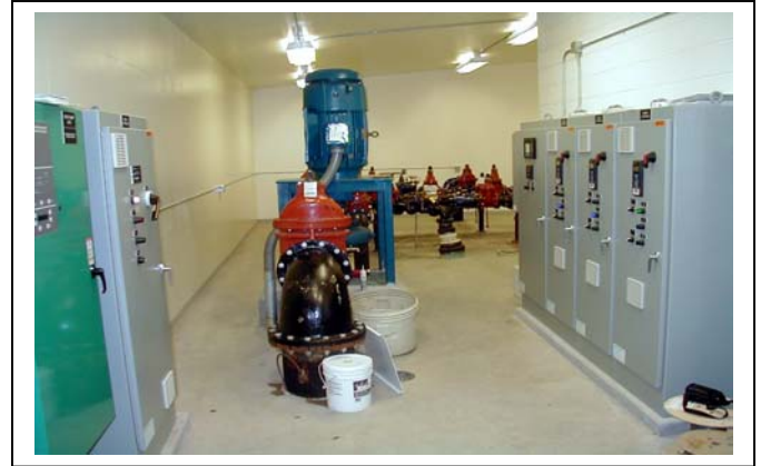
University Pump Station Interior with Controls and 200hp Pump. UAS Booster Station, Juneau, Alaska.
