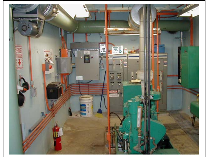
Allen-Bradley SLC RTU for Wastewater Pump Station No. 4. Ketchikan, Alaska.
