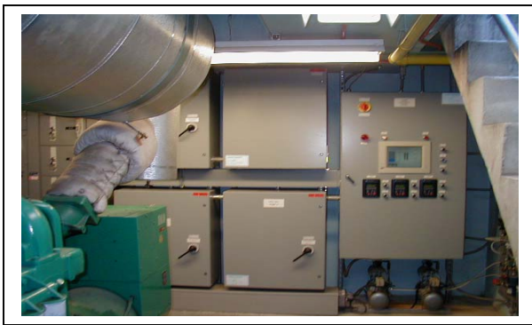
Wastewater Pump Station No. 2 VFD and PLC control panels. Ketchikan, Alaska.
