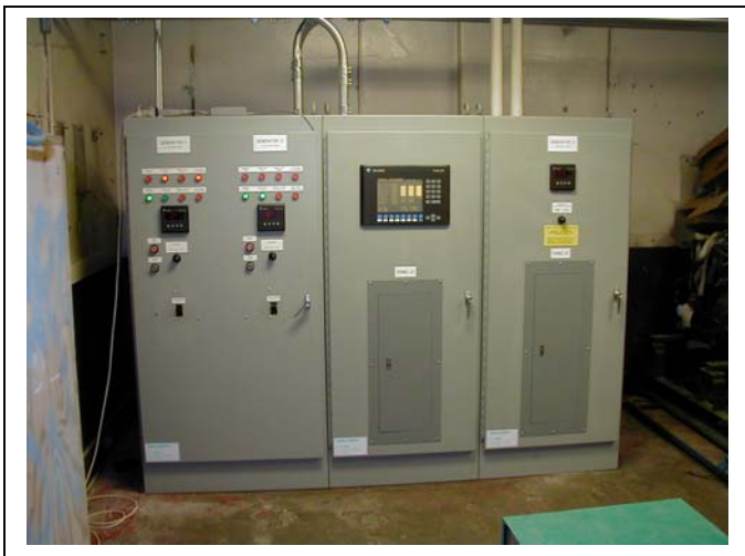
Generator Controls and SCADA Panel. Cape Hinchinbrook Light Station, Alaska.
