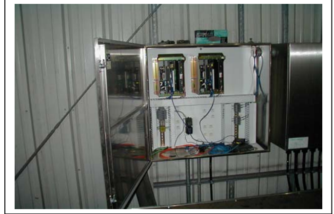
Hot Back-up Allen-Bradley PLC 5 control panel.
