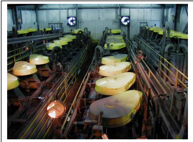
Zinc and lead flotation cells in Greens Creeks new cleaner flotation plant. Greens Creek Mine, Admiralty Island, Alaska.
