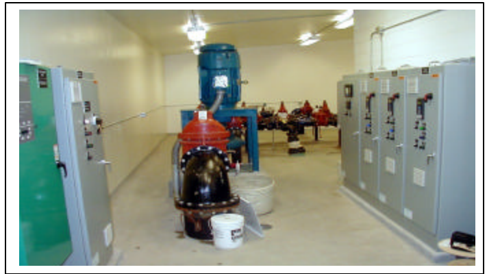
University Pump Station Interior with Controls and 200hp Pump. UAS Booster Station, Juneau, Alaska.
