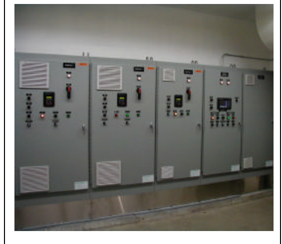
Outer Drive Pump Station Control Panels. Juneau, Alaska.
