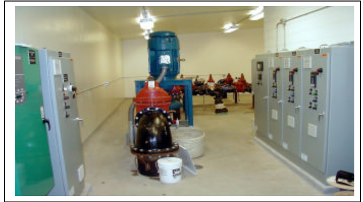
University Pump Station Interior with Controls and 200hp Pump. UAS Booster Station, Juneau, Alaska.
