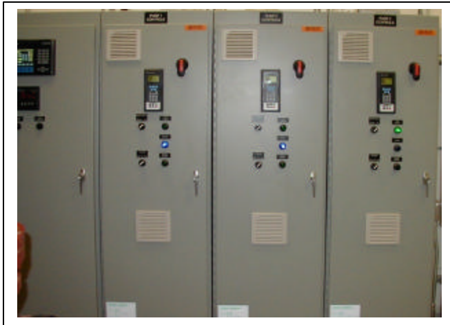
PLC Control Panel with Three 15hp VFD cabinets. UAS Booster Station, Juneau, Alaska.
