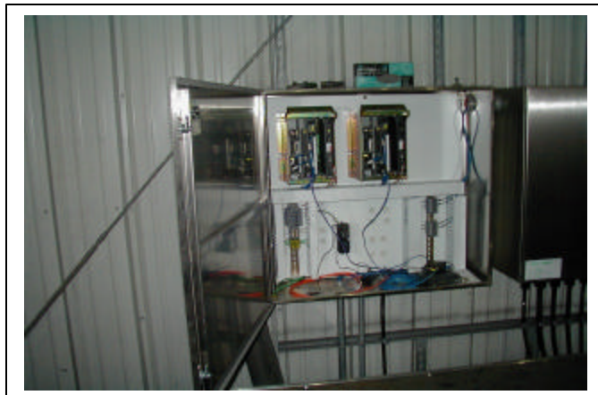
Hot Back-up Allen-Bradley PLC 5 control panel.
