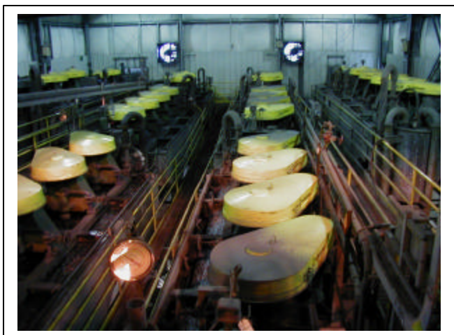
Zinc and lead flotation cells in Greens Creeks new cleaner flotation plant. Greens Creek Mine, Admiralty Island, Alaska.
